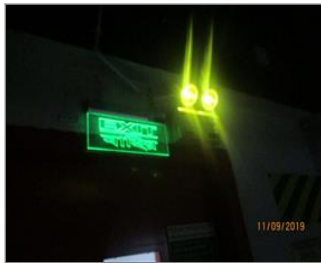
External photo(s) of the production unit(s) Emergency light check.JPG
