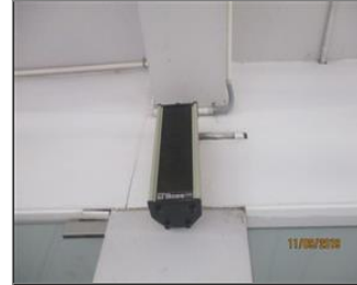
External photo(s) of the production unit(s) PA System.JPG
